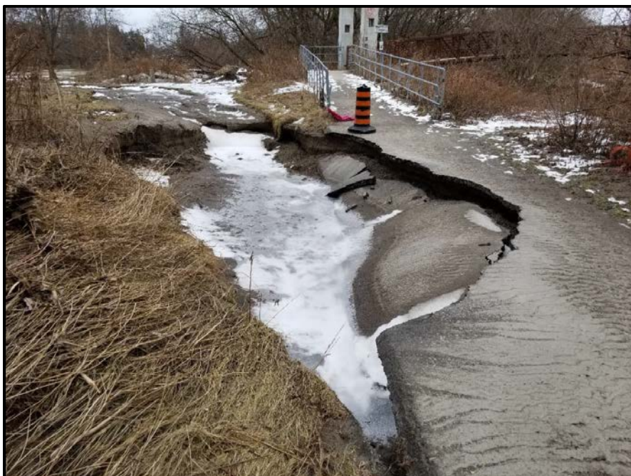
Figure 7 – Trans Canada Trail washout at Church Street and Highway 401
