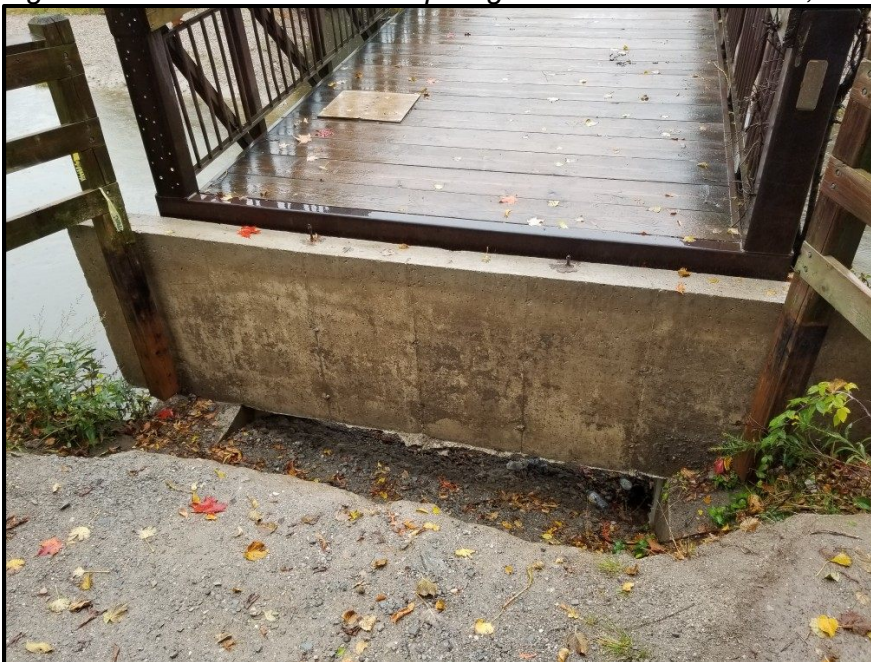
Figure 3. View of south pedestrian bridge embankment and large erosion scour
