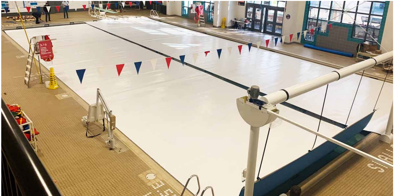
Figure 6: Pool cover installed at Ajax Community Centre.
