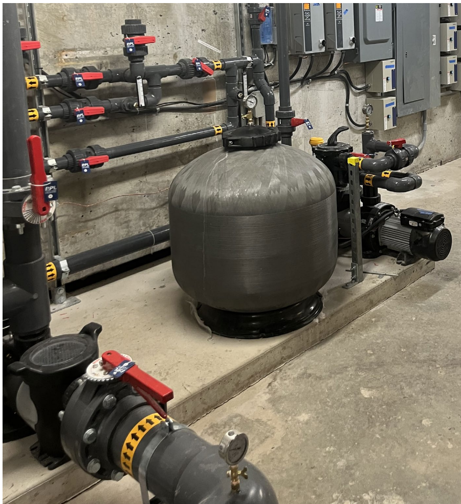
Figure 7: The new pool filtration system with VFDs and automated controller installed in the mechanical room of Mclean Community Centre.
