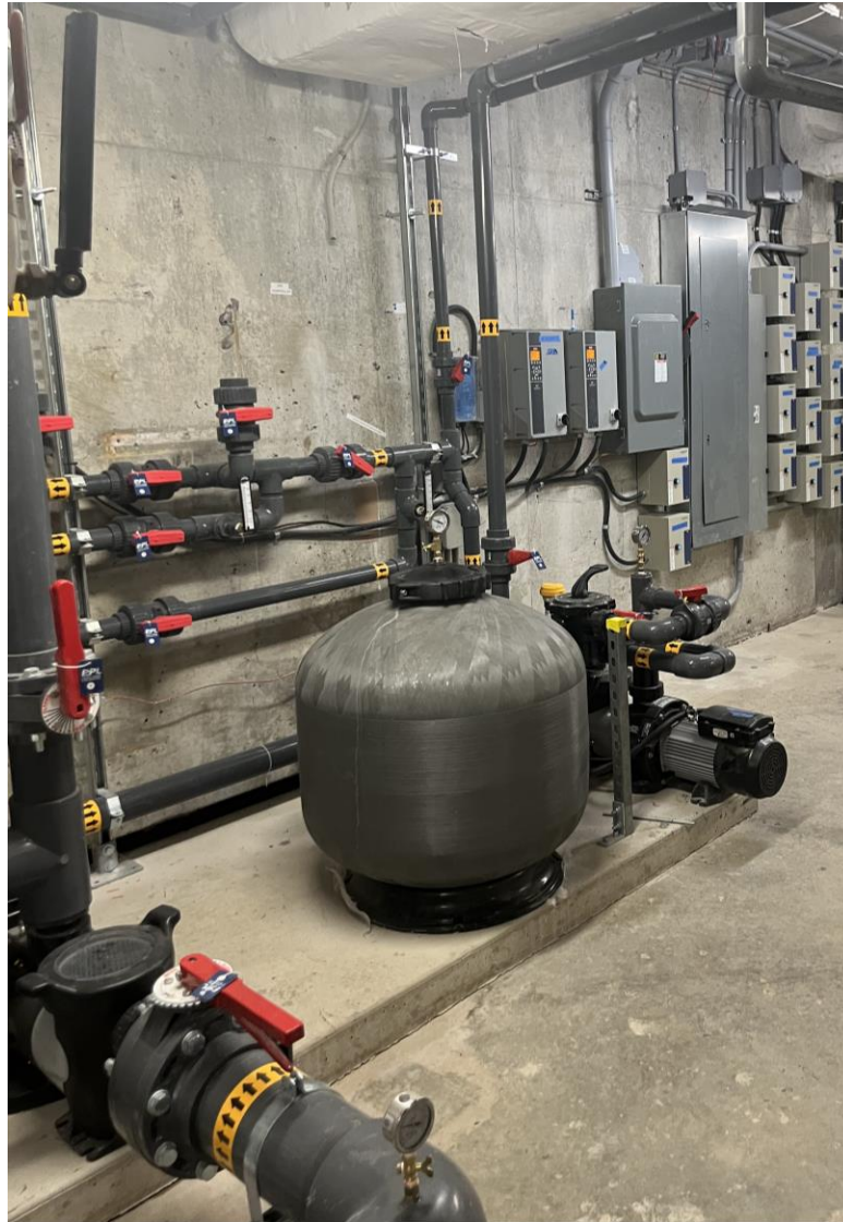
Figure 5: The new pool filtration system with VFDs and automated controller installed in the mechanical room of MCC.
