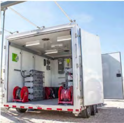
Figure 23 - Mobile DC Power Trailer (HM Cragg)
