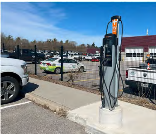
Figure 1 - ChargePoint Level 2 Charging Station at Town of Ajax Operations Centre
