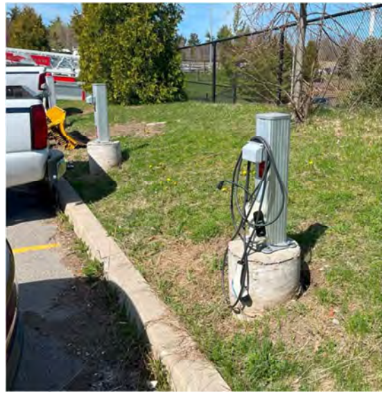
Figure 26 - Existing Level 1 EV Charging Cable at Operations Centre, April 2024
